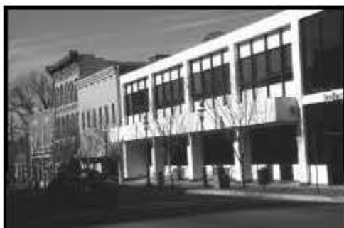
The color, materials and architectural detailing on the facade of this infill building are incompatible with the adjacent, older buildings.
