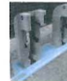
Non-bolted solar base plate
