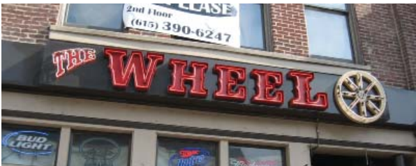
Example of raceway incorporated as sign background
